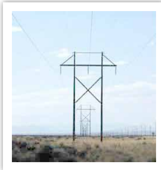
Double pole structure
