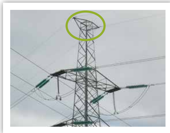
Ground conductor at the top of an HV transmission pylon
