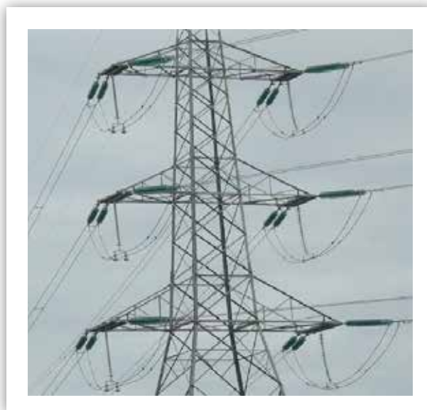
Transmission line carrying alternating current (AC) in two three-phase circuits
