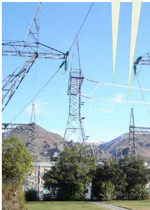
Support structure carrying direct current (DC)
