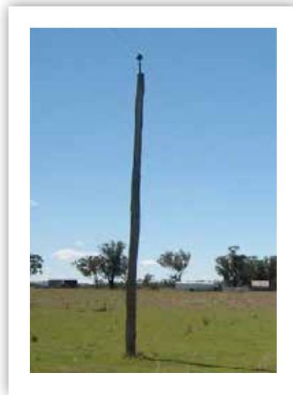
SWER – Single conductor and insulator on a pole
